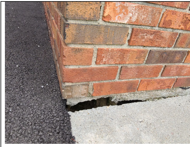
3. Damaged foundation located at the northeast corner of the structure
